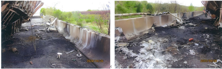
Fig. 19 Damage to existing bridge guardrails
