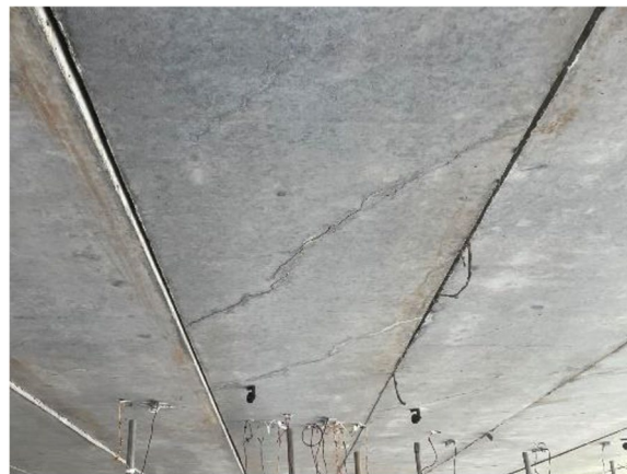
Fig. 2 Diagonal cracks at the bottom of slabs
