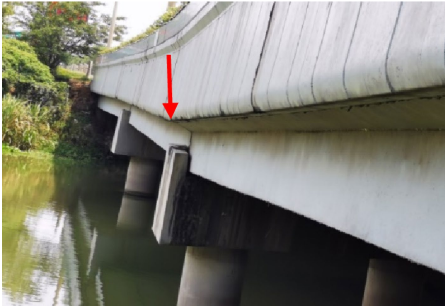
Fig. 10 The facade of pier #23 had a downward folding phenomenon
