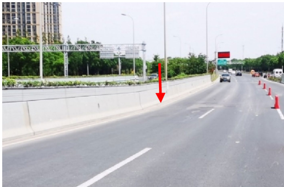
Fig. 9 The bridge deck on the west side of pier #23 had obvious depression
