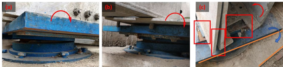
Fig. 11 Damage to bearing B1: a bearing under the left truss with significant rotation, b bearing under the middle truss with significant rotation, c bearing under the right truss with significant rotation as well as torsion about vertical axis
