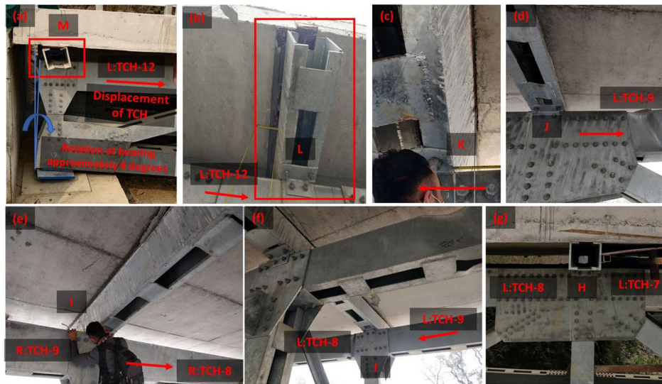
Fig. 6 Observed damage in top cross beam: a joint M, b joint L, c joint K, d joint J, e joint I at right truss, f joint I at left truss, and g joint H
