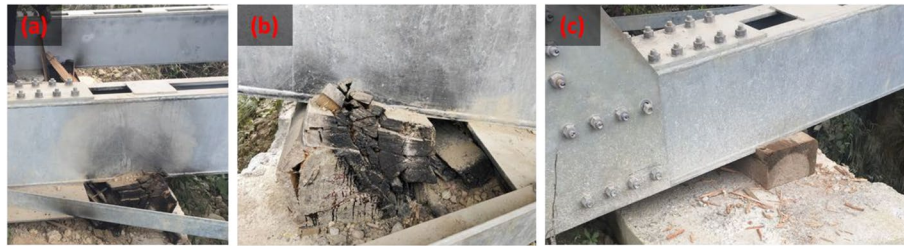
Fig. 36 Temporary supports at X: a under the middle and left trusses that were crushed after burning, b close up view of temporary support under middle truss, c restored temporary support under right truss
