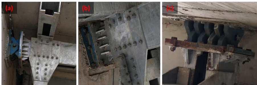
Fig. 14 Steel hinge bearing A1: a side view, b oblique view, c bottom view
